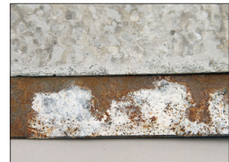
Figure 5– Galvanic corrosion can occur between dissimilar metals if precautions are not taken.
